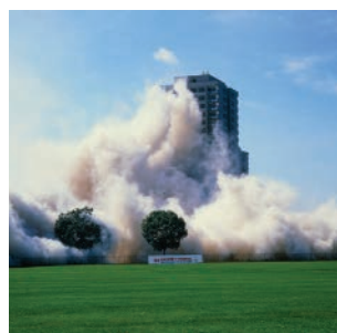
▲ Figure 16.2 Explosives produce large quantities of high-pressure gas. When the gas expands, it does work in demolishing the building.
