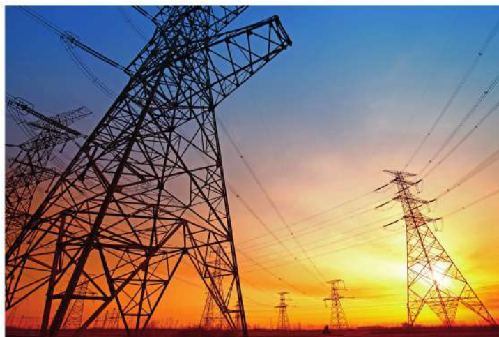
▲ fig A Transmission lines can carry very high voltages, generating significant electric fields.
