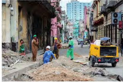
▲ Figure 21.9 Transportable generators are used to produce electricity for the lights and machinery used on roadworks.
